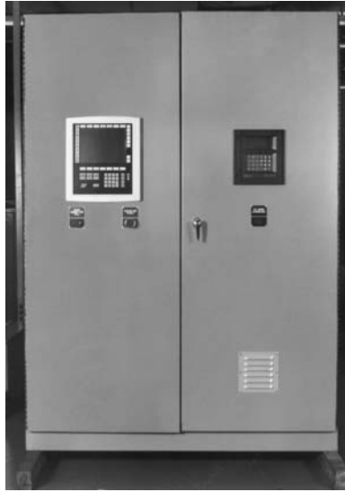
FIGURE 21.6 Pipeline compressor panel (programmable logic controller and temperature scanner) front panel view. (Courtesy of Advanced Control Engineering Services).
