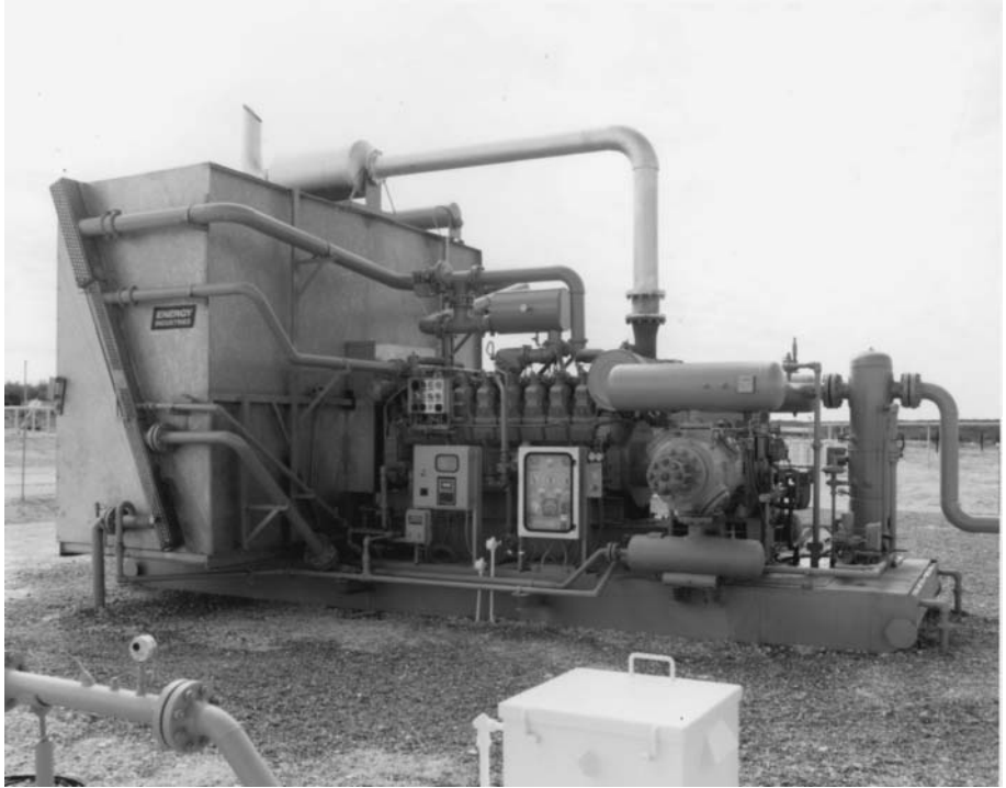
FIGURE 23.11 Typical reciprocating unit, CAT G3516LEA/FE665-21, Energy Industries.
