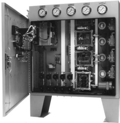
FIGURE 21.2 Nitrogen Compressor Control Panel (Class I, Group C & D, Division II Area) inside panel view. (Courtesy of Autocator Products Division T. F. Hudgins, Incorporated).
